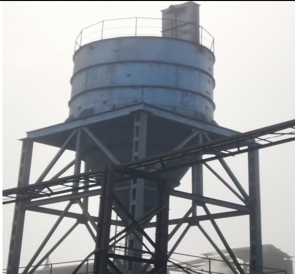
Ash silo dust collection installed in DRI cooler discharge area kiln #03
