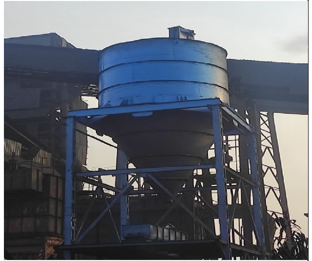
Ash silo dust collection installed in product hopper bag filter area
