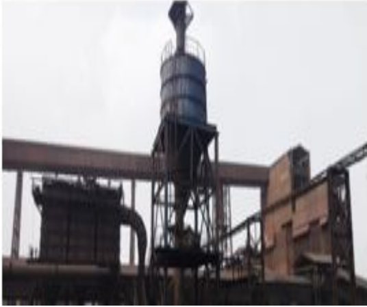
Ash silo dust collection installed in DRI cooler discharge area
